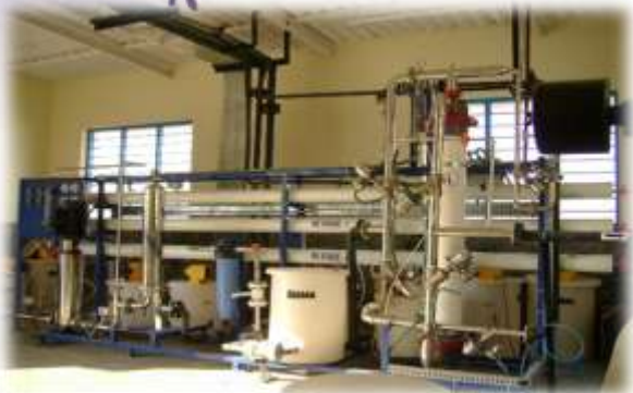
View Of Ultra Filtration Plant at Sierra Silk
